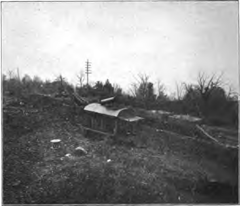
Excavation on Belleville turnpike, Bergen Co. This is where we are getting our filling. Showing the steam shovel and engine for hoisting the cars from the bottom of the hill.
